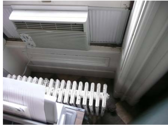
Window AC Unit at Office 102
