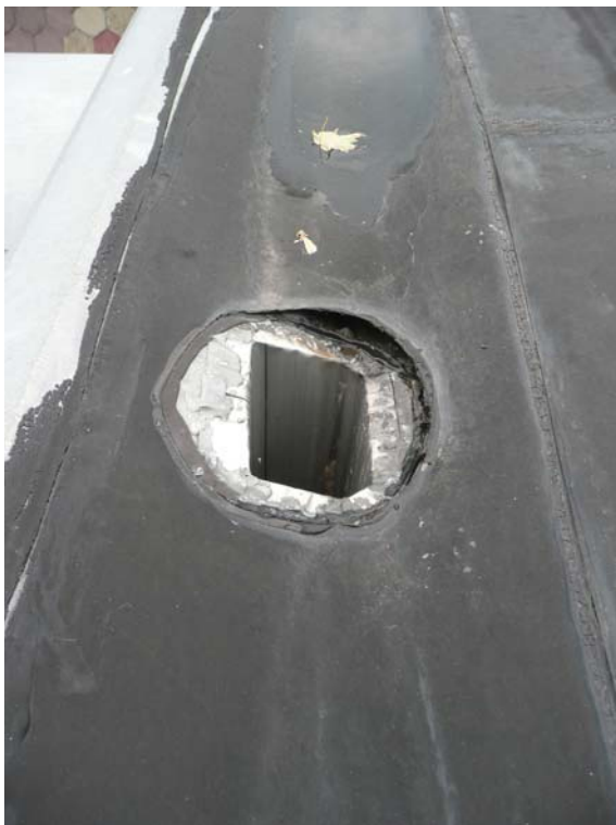
Failed EPDM Roofing at Downspout (Typical)
