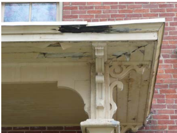
Detail of Damaged Wood from Leaking Roof
