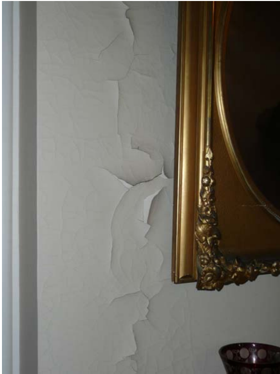
Deterioration of Wall Finish at Fireplace
