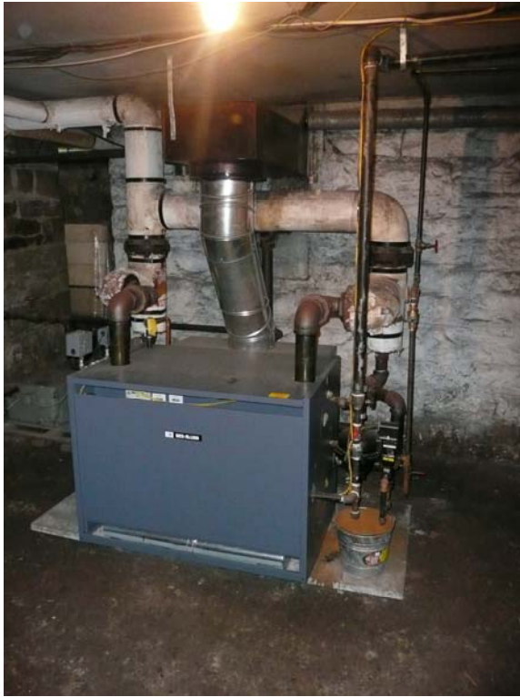
View of Steam Boiler
