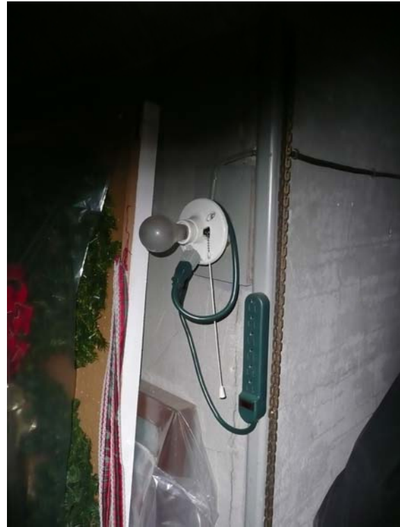
Detail of Lighting and Electrical
