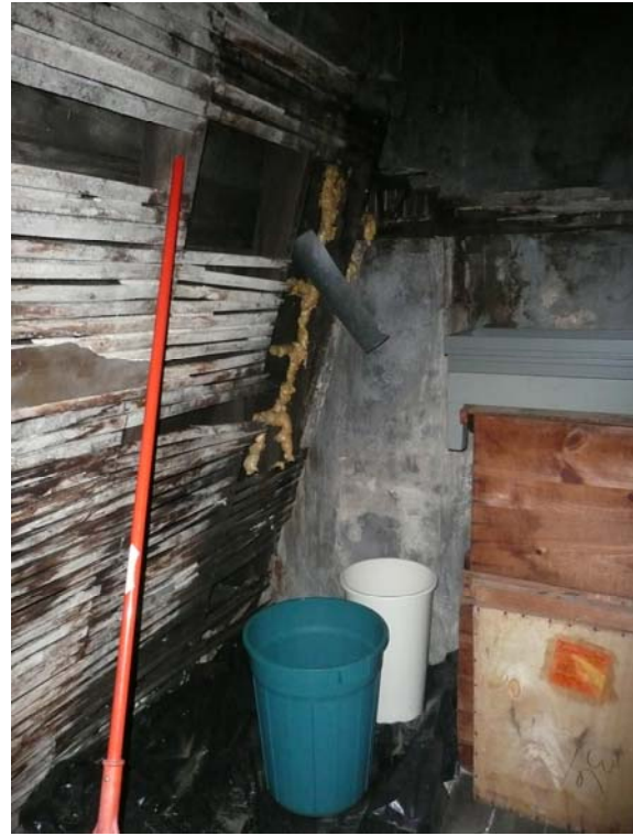
Detail of Southeast Corner with Water Damage
