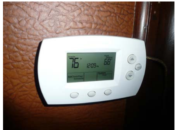
Programmable Thermostat in First Floor Stair Hall
