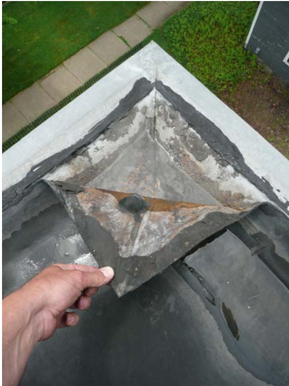
Failed EPDM Roofing at Southwest Corner of Front Roof
