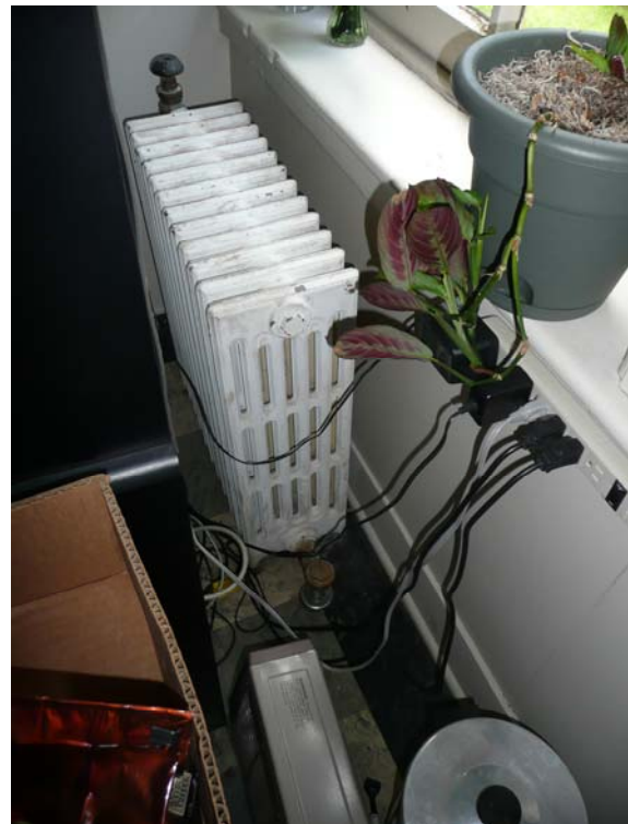
Electrical Wiring at Archive Storage 107
