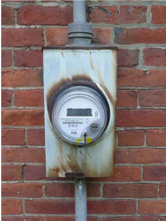
Electric Meter at North Side of Building
