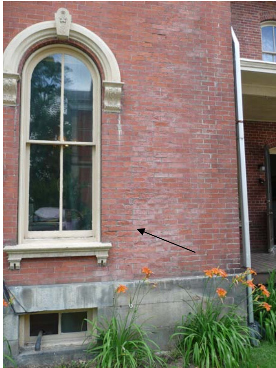
Damaged Brick at East Elevation (arrow)
