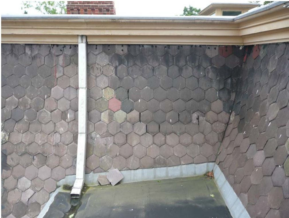
View of North Side (east) of Front Roof Showing Original Slate and Downspout from Flat Roof
