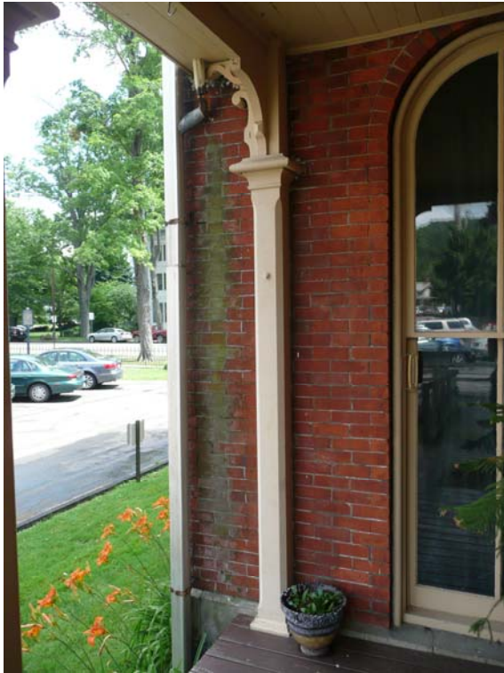
Detail of Porch – Downspout Leaking on Brick
