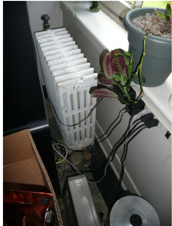
Typical Cast Iron Radiator
