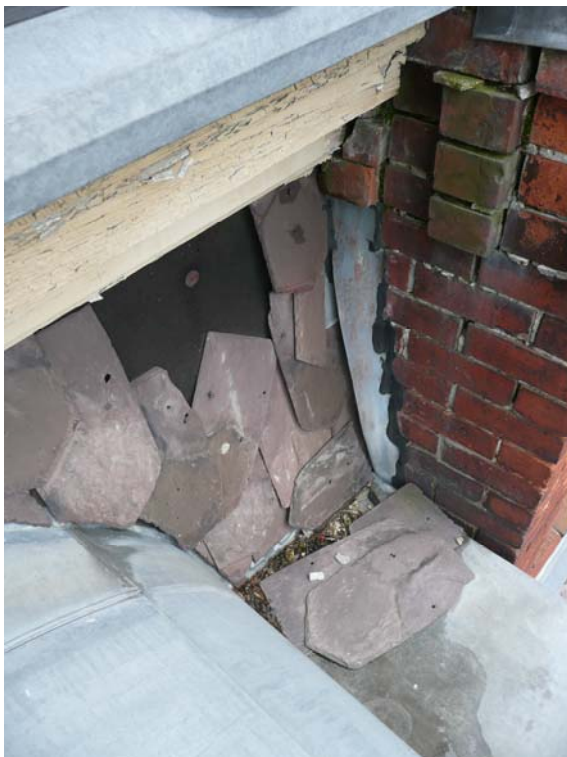
Damaged Slate North of West Chimney
