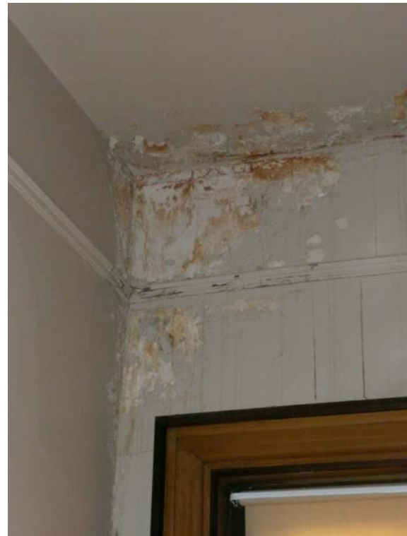
Detail of Water Damaged Plaster at West Wall
