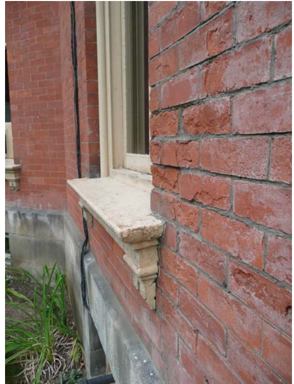
Detail of Damaged Brick at East Elevation
