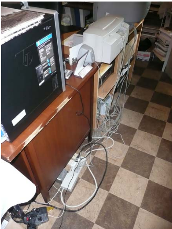
Electrical and Data Wiring at Office 102
