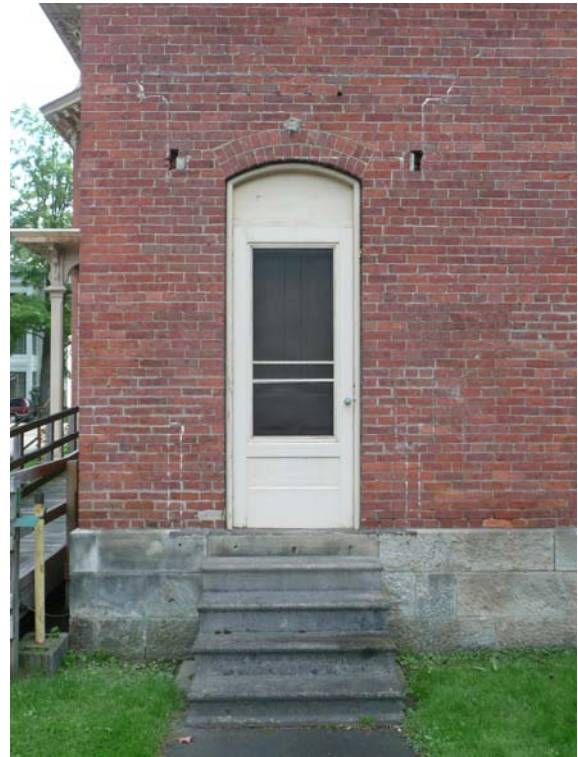
North Entrance with Evidence of Missing Projecting Covering and Railings
