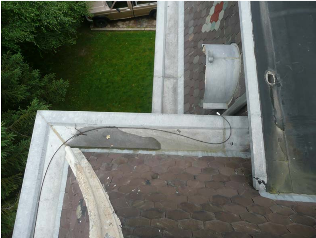
View of West Side of Intersection of Front and Rear Roofs looking North
