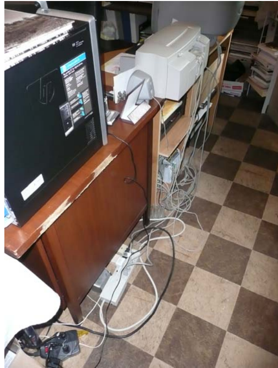
Electrical and Data Wiring
