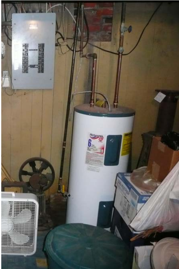
Electric Hot Water Heater at Room B05
