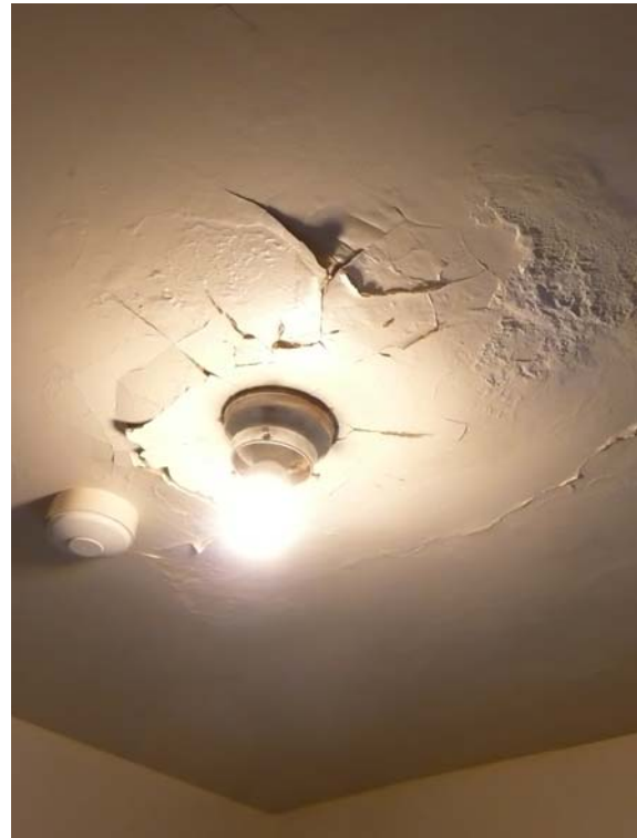
Light Fixture with Plaster Damage at Restroom 211
