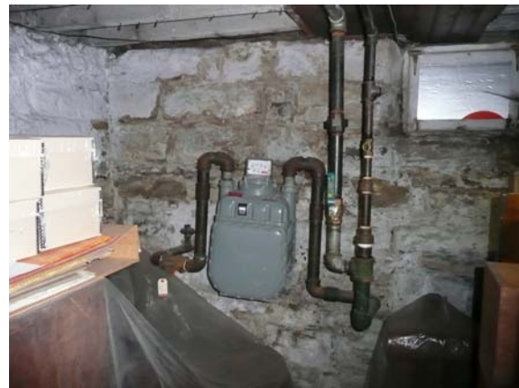
Gas Meter at South End of Room B03
