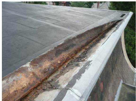
Failed EPDM Roofing at North Edge of Front Roof
