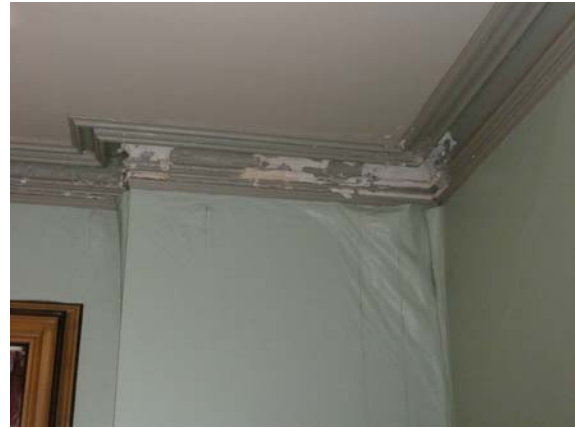
Detail of Water Damaged Plaster at Chimney
