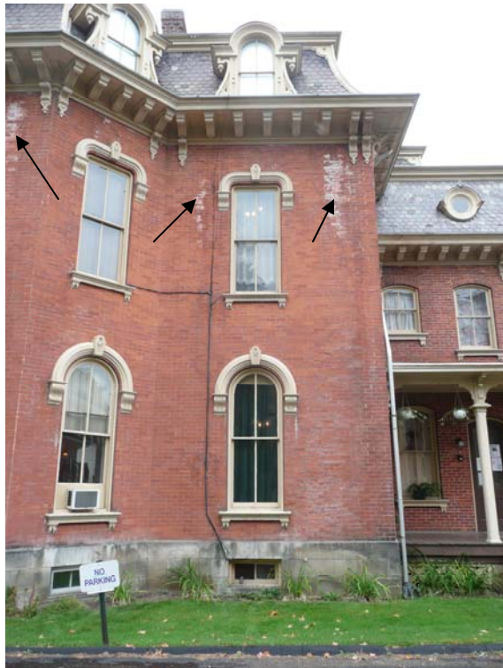
Efflorescence on Brick (arrows)
