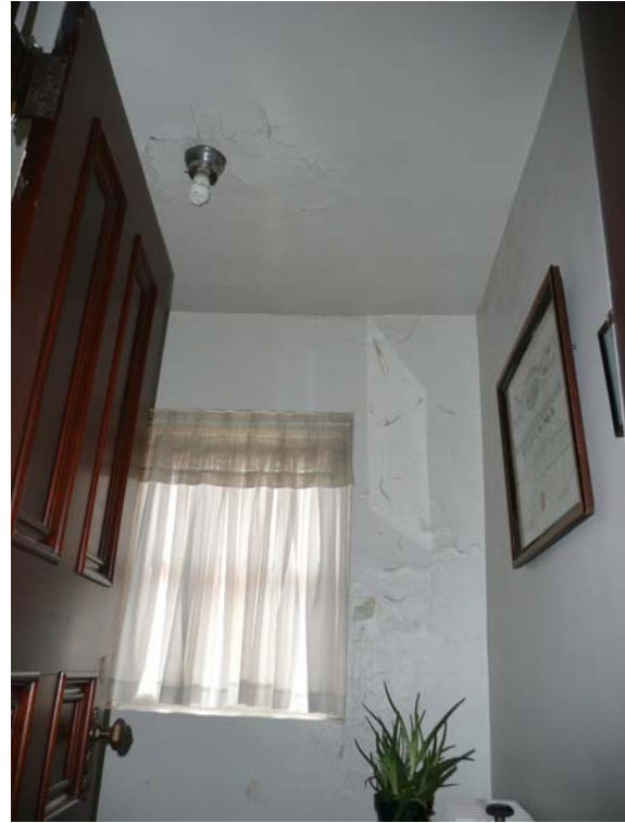
View Looking East at Water Damaged Plaster
