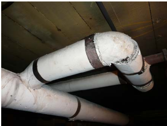
Insulation on Steam Heating Pipes
