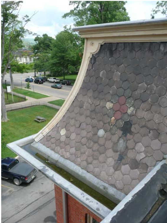
View of North Side (East) of Front Mansard Roof (Note standing water in gutter and incorrect repair of missing slate)
