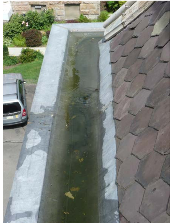
Plugged Downspout at Northeast Corner of Front Roof
