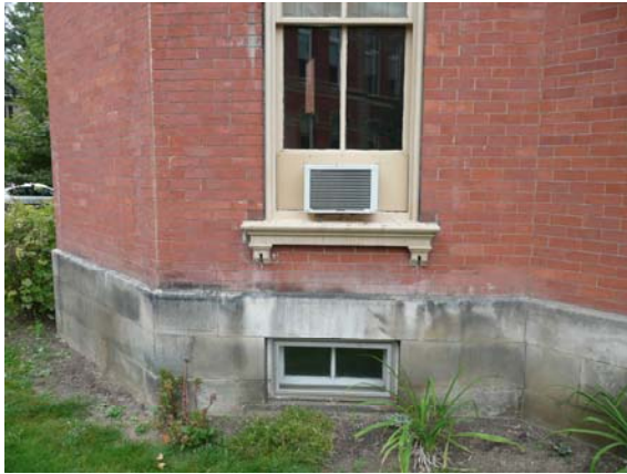
Window AC Unit at Office 102
