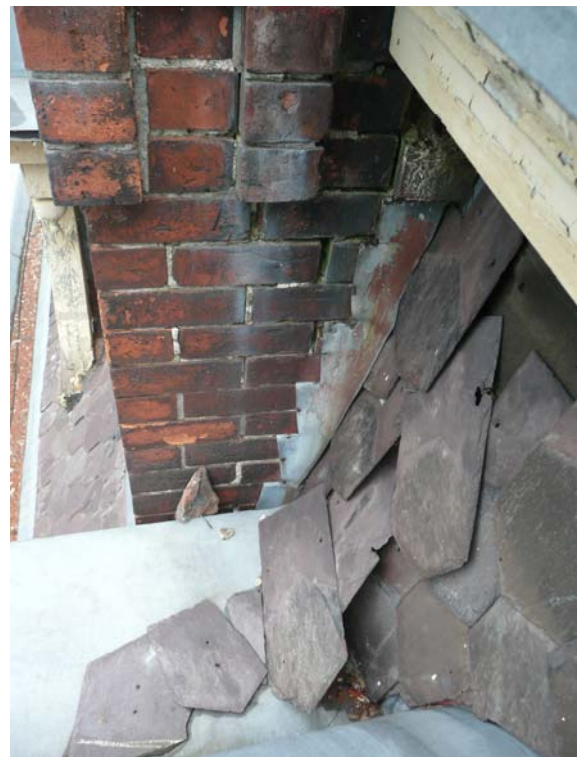
Damaged Slate South of West Chimney
