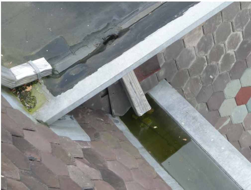
Detail of Gutters at East Side Intersection of Front and Rear Roofs (Note loose slates and standing water. This is the location of an active water leak inside building)
