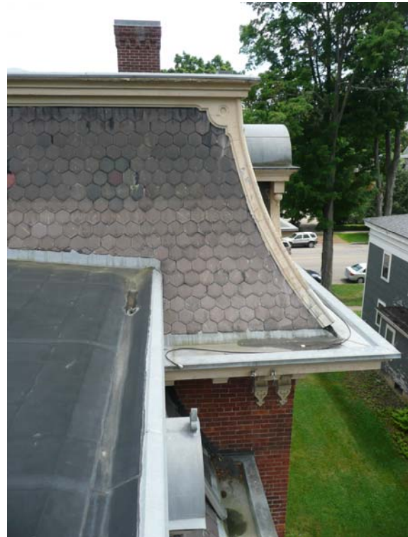
View of North Side (West) of Front Mansard Roof (Note heat tape in gutter)
