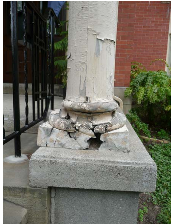
Detail of Deteriorated Column Base
