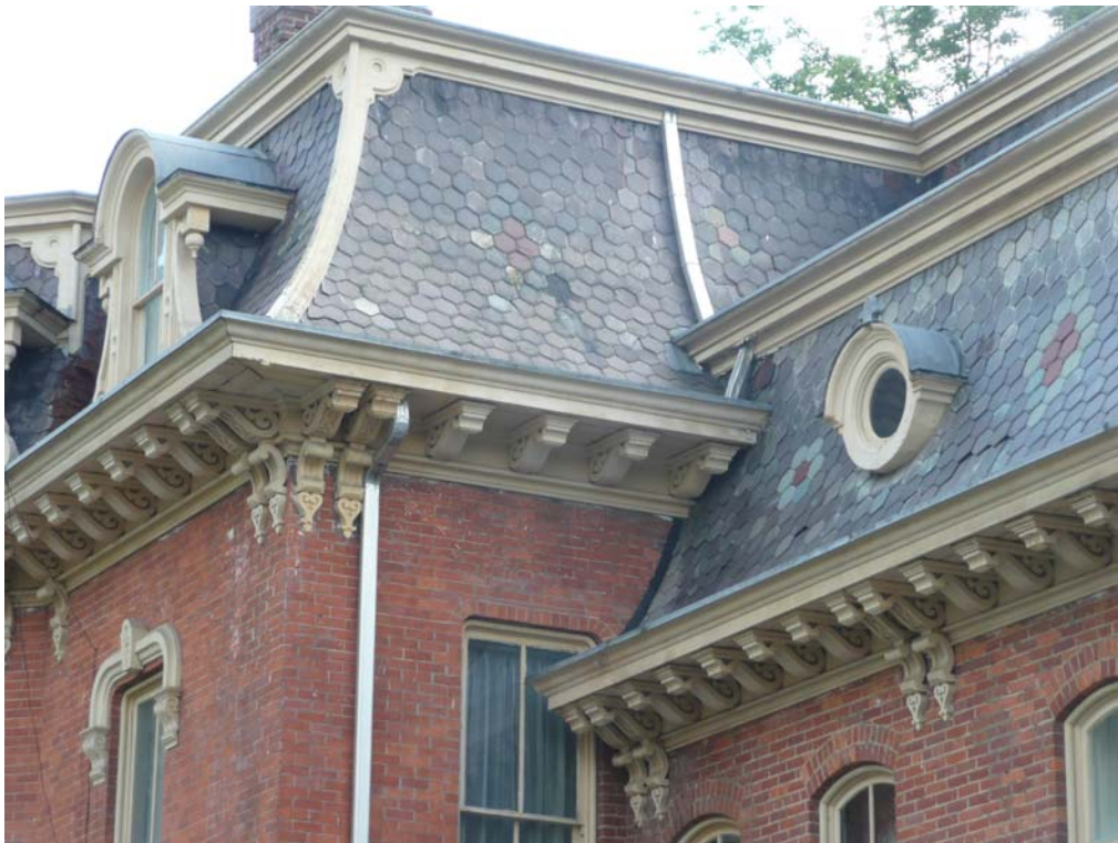
Typical Upper and Lower Cornices at Mansard Roof (Northeast corner of front mansard roof)
