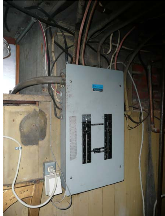
Main Electrical Panel
