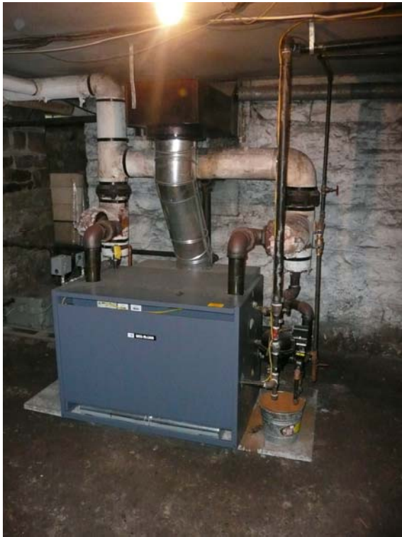
Steam Boiler in Boiler Room B07
